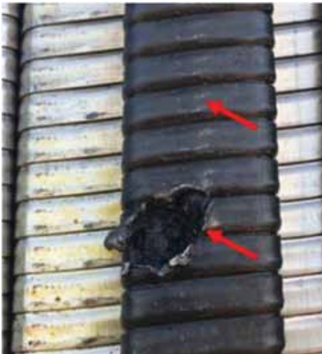
Figure 5—Burned cable adjacent to pump (notice the wear mark indicates the contact line to ESP string)
