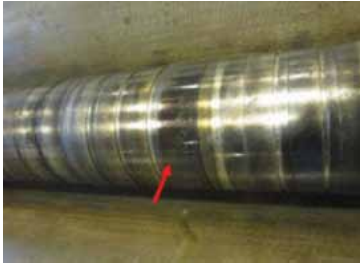
Figure 2—Heat discoloration on diffusers
